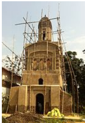
The entrance to Kedamath Datta's maternal home in Birnagar (Ula), West Bengal under renovation. 2014
